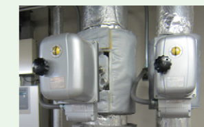
Steam supply is automatically controlled through a valve
