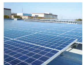
Solar panels at the Shiga factory
