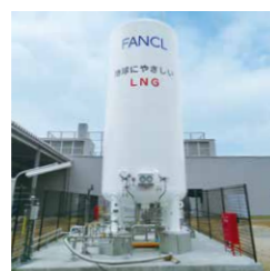
LNG tank at Shiga Factory (refilled with carbon-neutral LNG from July 2022)
